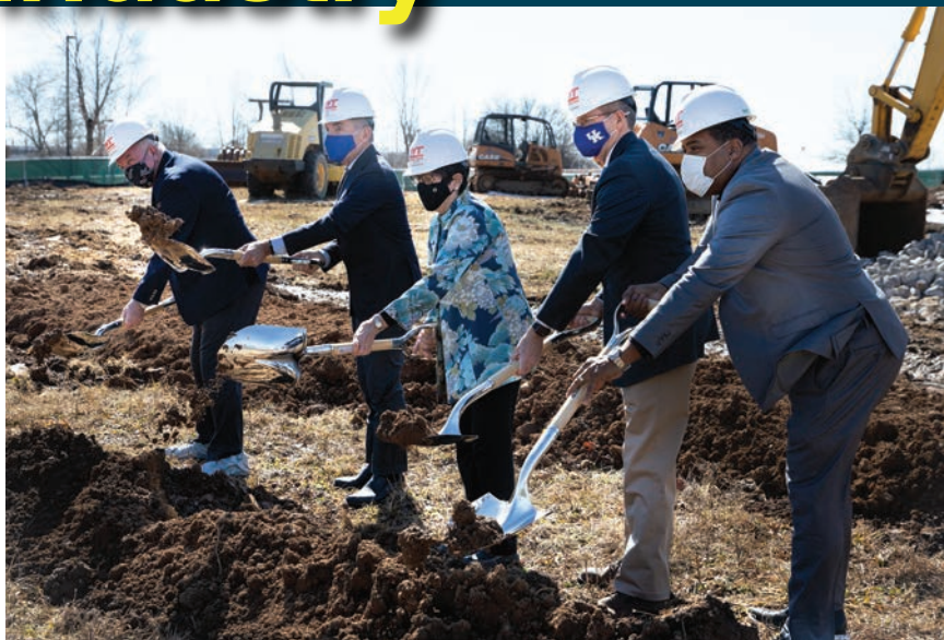
Groundbreaking for The Core, which is the University of Kentucky's new development for early-stage, high-tech companies due to be completed in 2022. (UK Photo by Mark Cornelison)
